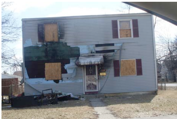
This house is burned out, vacant and left to decay on the East side of Columbus.
